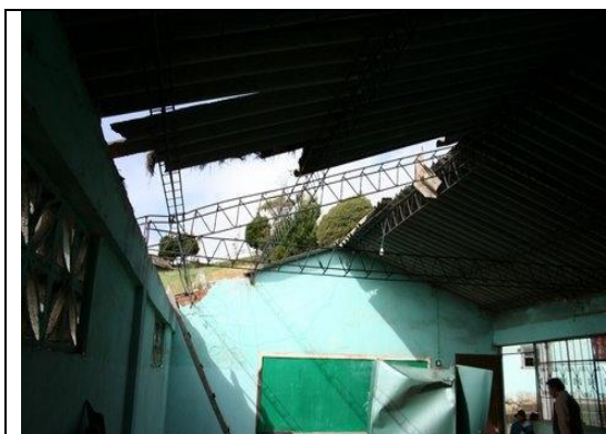
Convalecencia's School ceilings destroyed by a tree that fell.
