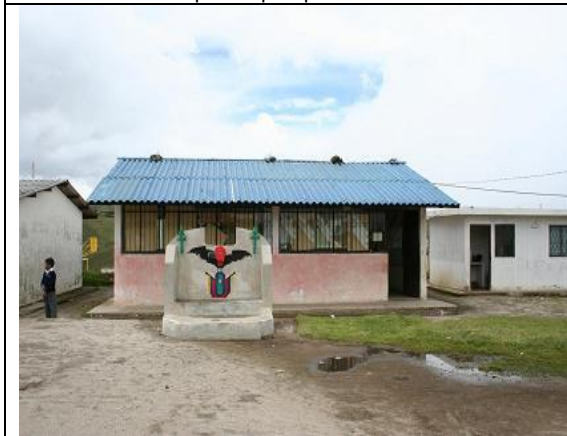
Classroom with old ceilings in Tupac Yupanqui's School
